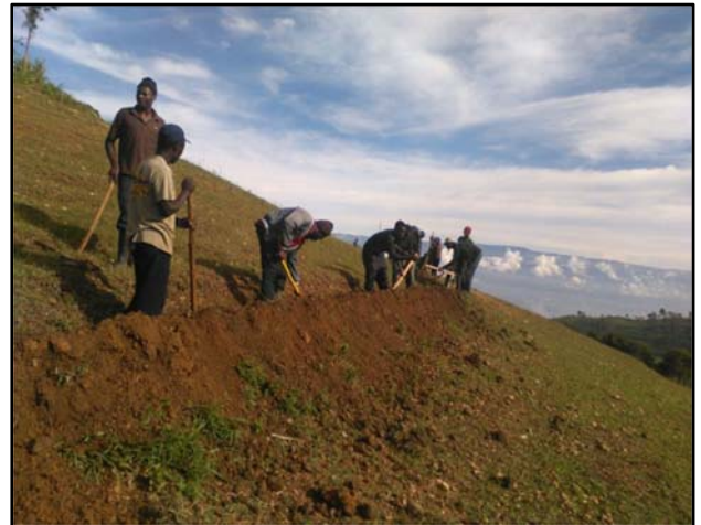
Soil and water retention system being built into a hillside in Boucan Chat. Credit: EPIC
